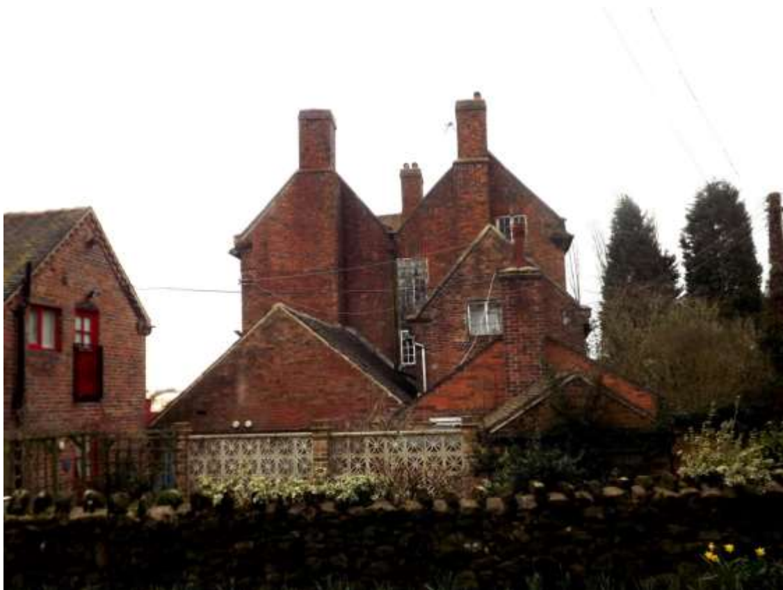
Figure 39 Parts of Fulford Hall have suffered from lack of maintenance and repair
