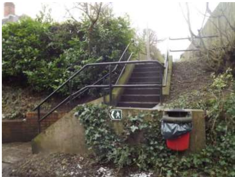
Figure 38 Concrete walls and steps, modern railings and signs detract from the character of the conservation area
